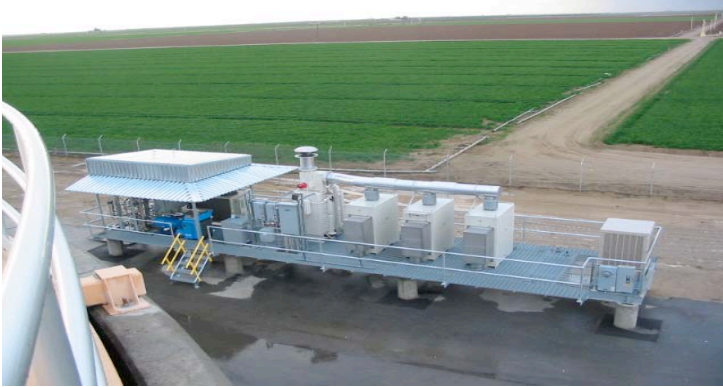
Biogas Fuel Conditioning Skid Example
