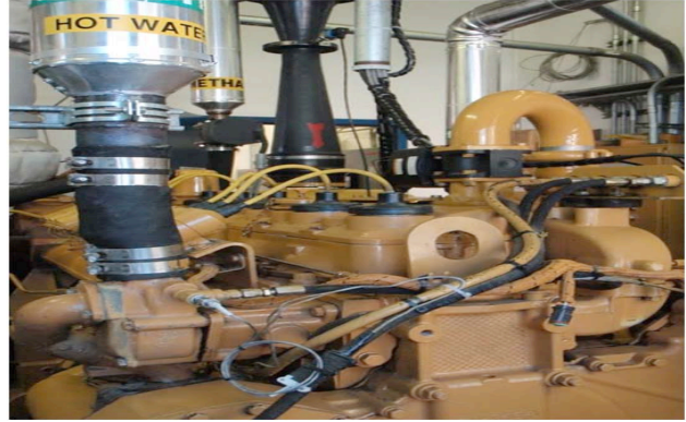
Generator at the Burlingame WWTP
