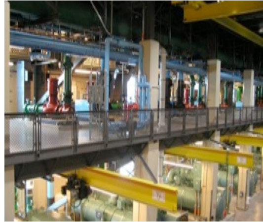
DGS Central Plant Chillers
