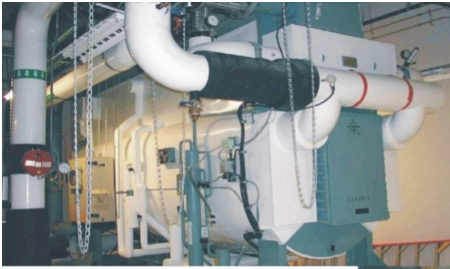
To left: 500 refrigeration ton (RT) absorption chiller
