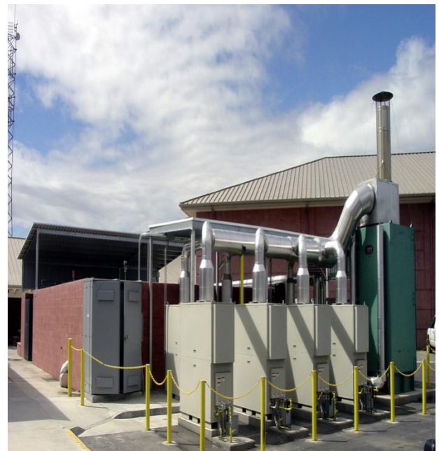
EMWD Capstone Microturbines
