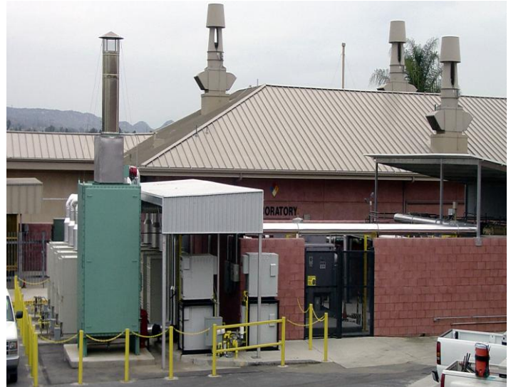
Heat Exchangers and NG Compressors
