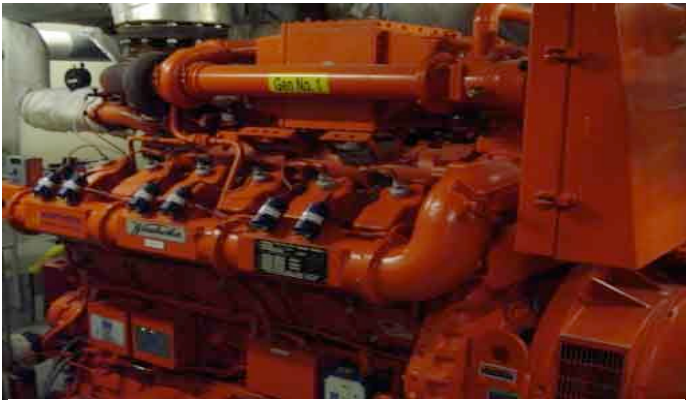
500 kW Waukesha VGF Generation Set
