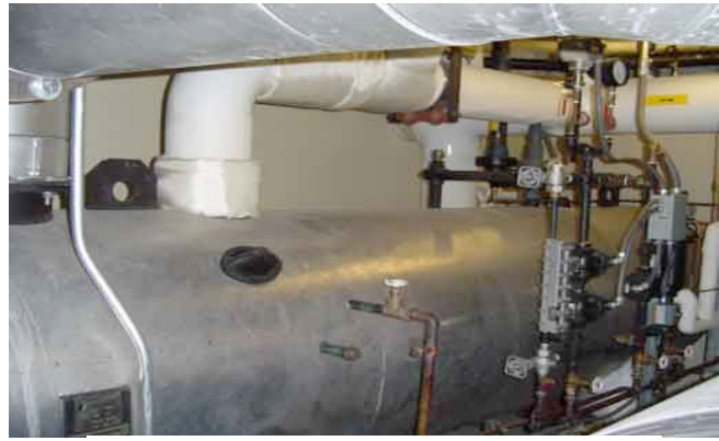
Heat Recovery Steam Generator
