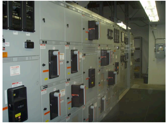
SFSU Central Plant Switchgear for CHP System
