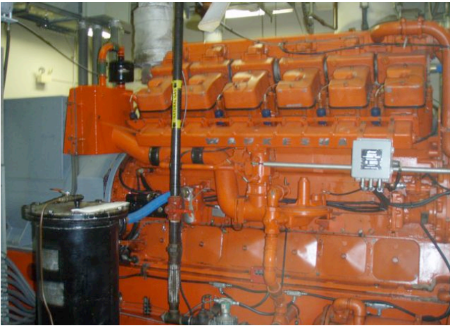
725 kW Original Waukesha Engine – 28 years of runtime!
