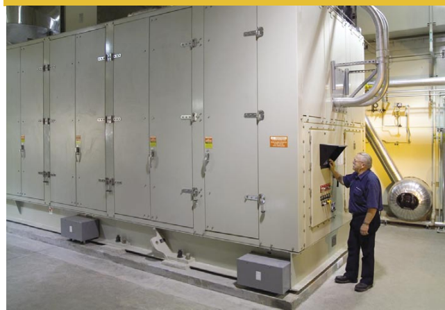
4.6 MW Mercury™ 50 gas turbine at SDVA
