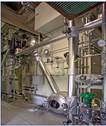
Gas turbine exhaust controls
