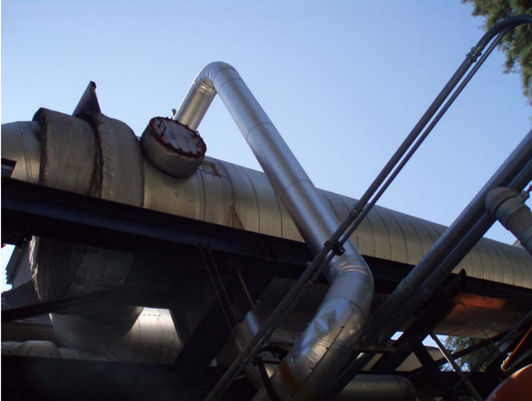
Figure 2: Heat Recovery Boiler
