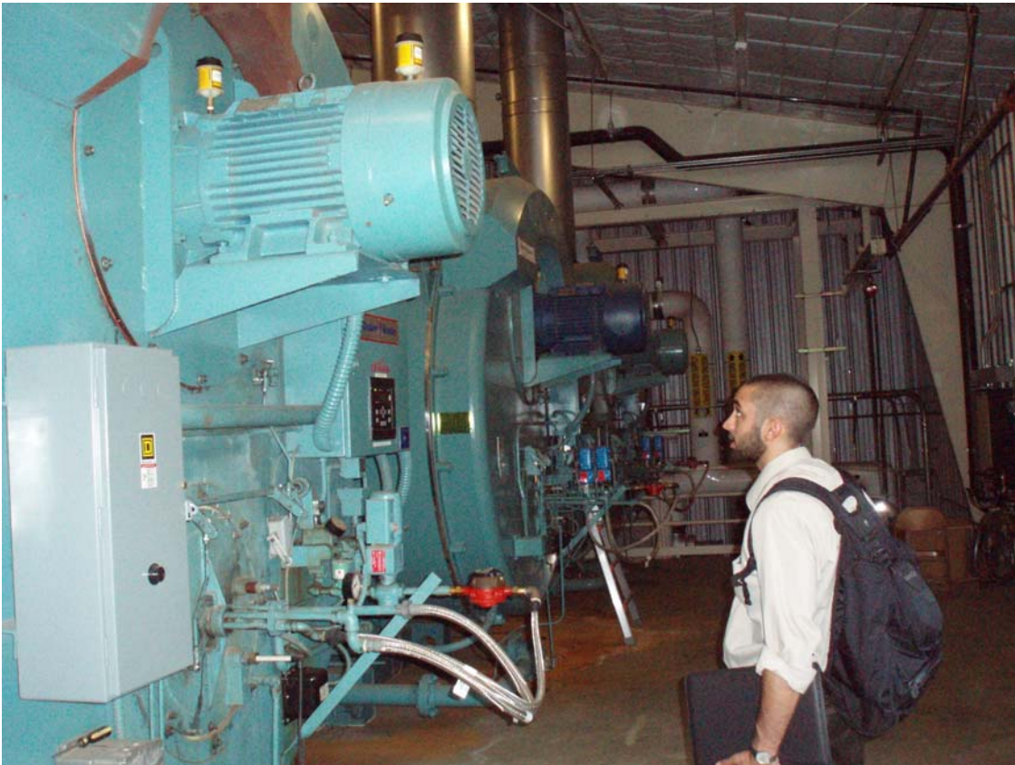
Figure 1: Three boilers currently providing hot water
